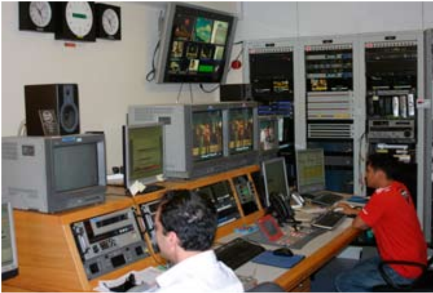
Operators working in the SAT-7 Master Control Room (MCR)
